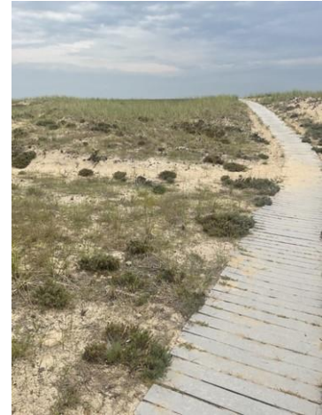
Figure 1: Bare sand strip perpendicular to walkway
